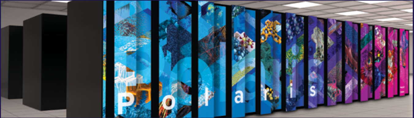
Polaris, a hybrid CPU-GPU system built by HPE, will help ready scientists for the arrival of the ALCF's Aurora exascale supercomputer.
