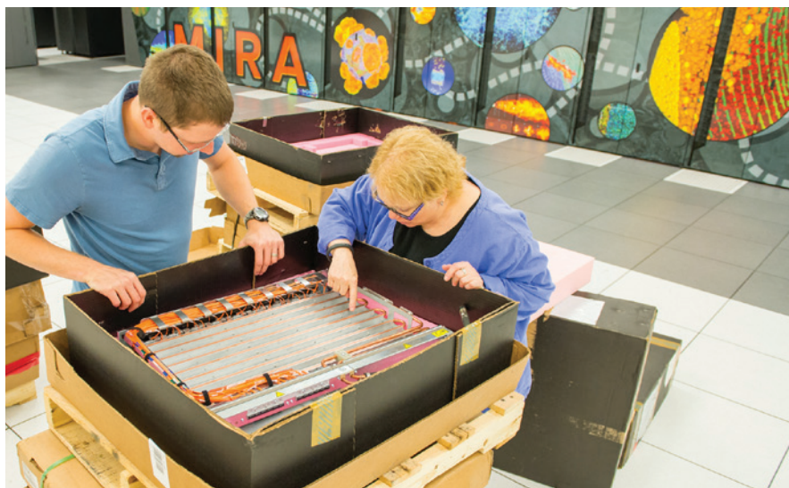
Susan Coghlan and Eric Pershey of ALCF discuss computing hardware in the facility's machine room.
